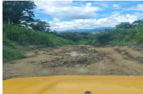
Deteriorated road leading to Utu SHC
