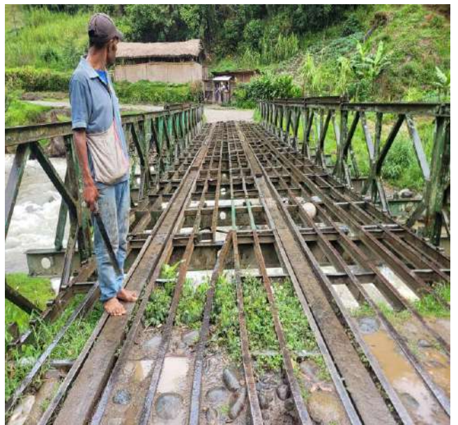
Dismantled bridge to Denglagu HSC. Timbers taken off and unable to pass through so turned back.
